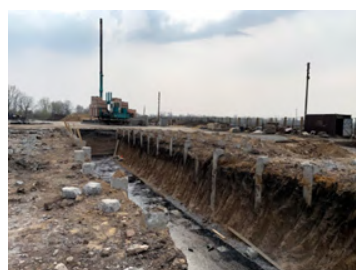
Figure 7. Strengthening of base by built-up reinforced concrete piles under foundation of silo with underground gallery in uts. Kov’yag of Kharkiv region.
