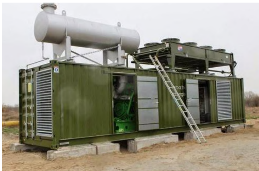
Figure 8. Jenbacher generator at the landfill in Zhytomyr with a capacity of 1 MW [34].
