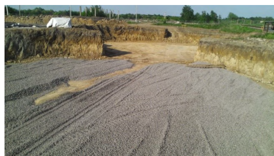
Figure 5. Arrangement of damper layer over reinforced base of silo by vertical soil cement elements in v. Velyka Doch, Chernigiv region.
