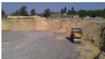
Figure 6. Arrangement of crushed rock cushion on sand soils under silo foundation in t. Shostka of Sumy region.
