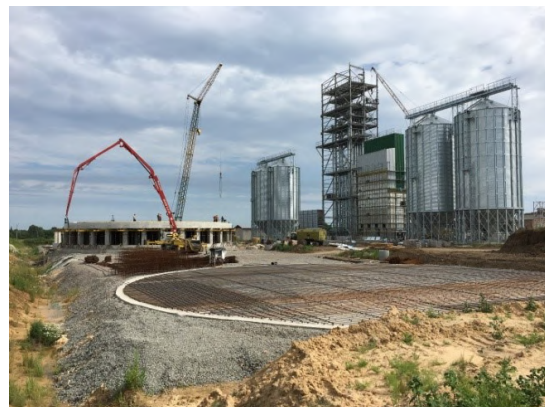
Figure 3. Arrangement of silo foundations on the base of strengthened soil in t. Krolevets’, Sumy region.
