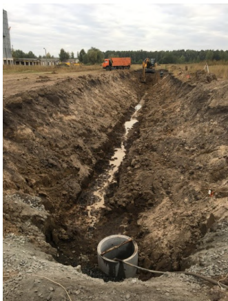
Figure 2. Water lowering before performing works on exploitation of pit and reinforcing silo base in t. Krolevets’ of Sumy region.
