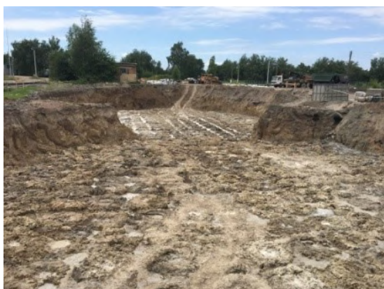
Figure 4. Strengthening of silo base by vertical soil cement elements in v. Velyka Doch, Chernigiv region.
