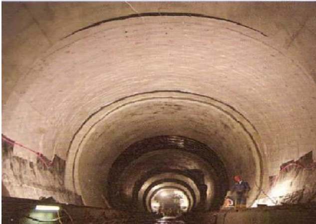
Fig. 2. Mounting of a manifold of thermal pumps within experimental area in Lainzer tunnel (Austria)
