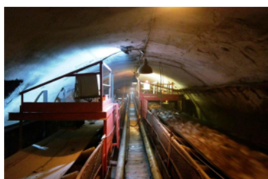
Fig. 3. OCS RLP-21T on conveyors No. 1A (right) ZhDM-1.
