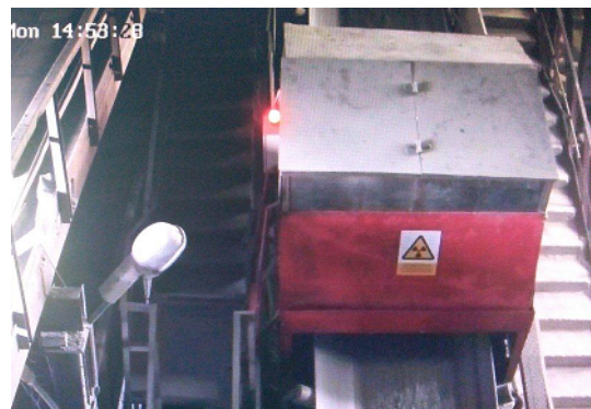
Fig. 5. OCS RLP-21T on conveyor No. 4 KPP.
